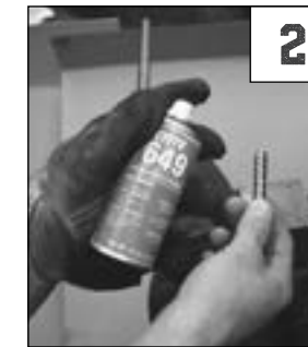
2. Spray Loctite Primer in and around the cable end and splice core to thoroughly remove grease and grime.
